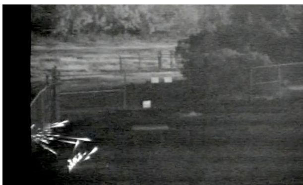
Surveillance footage released by PG&E shows the sparks from bullets hitting the substation equipment.
